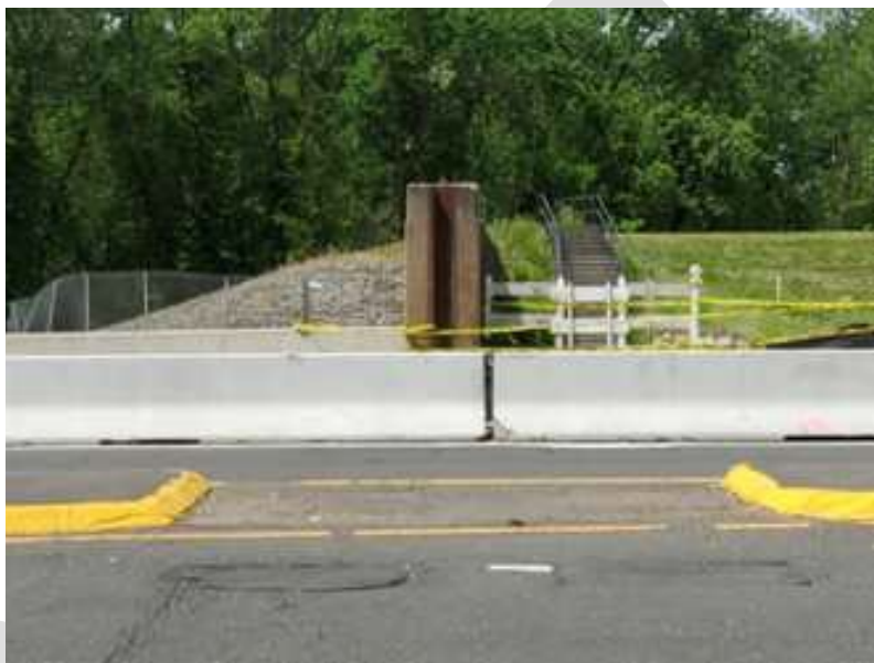
Figure 39: Site Potential Seepage at the Steps of the Main Street Closure
