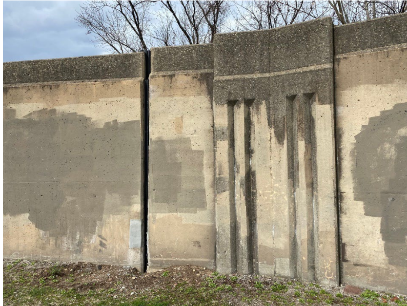
Figure 36: An Example of a Concrete Floodwall Located at Dutch Point in Hartford, CT
