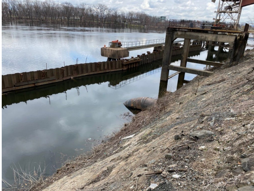
Figure 51: The Riverbank slope at the Materials Innovation and Recycling Authority Site
