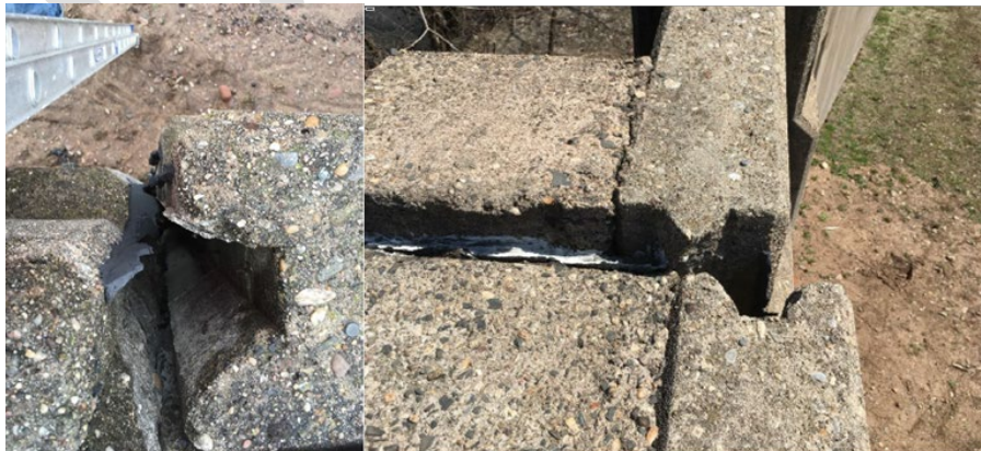
Figure 72: Joint Displacement at the Dutch Point Flood Wall Location, Hartford
