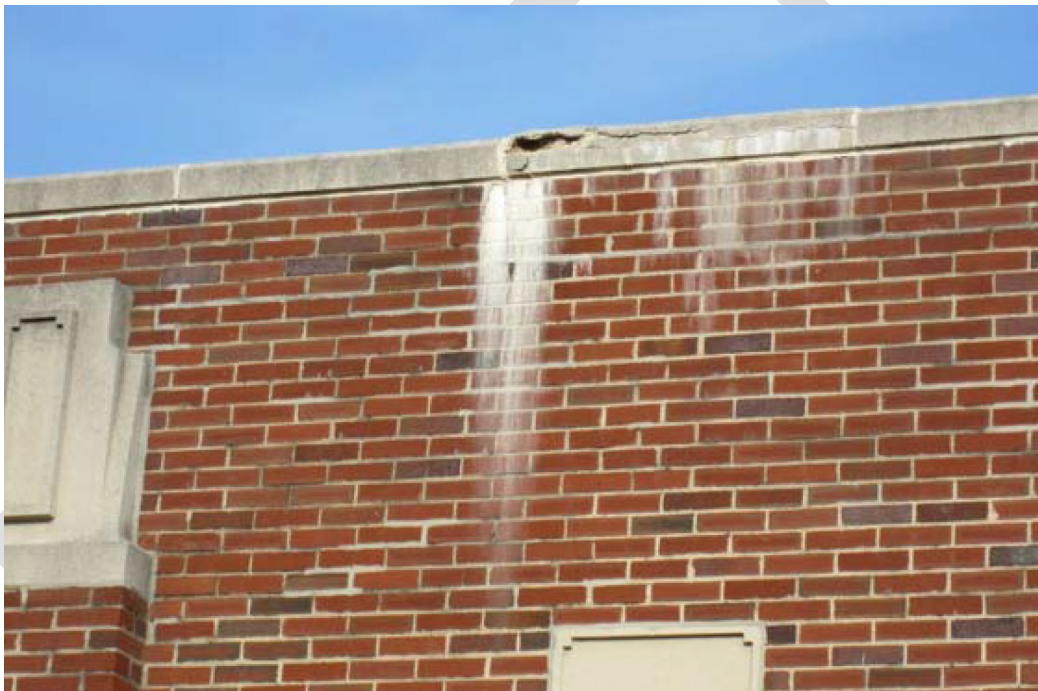
Figure 36: Detail of Damaged Concrete on the Rook of the South Meadows Pump Station
