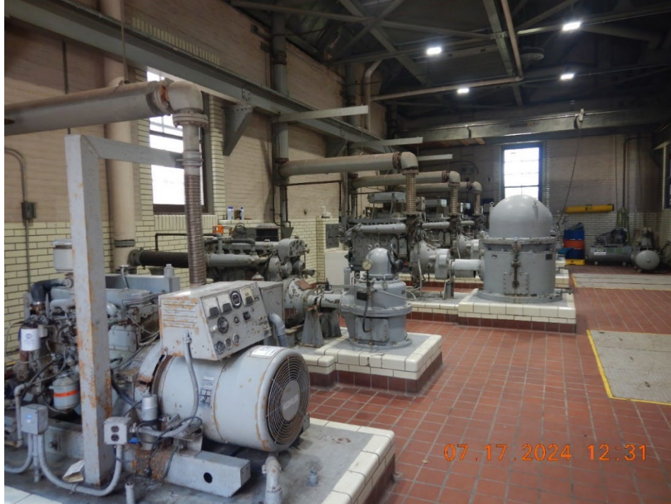
Figure 46: Motors for Five Pumps at the Bushnell Pump Station
